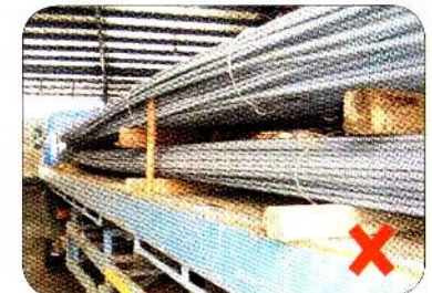
Bundles of steel rods are not properly secured.
